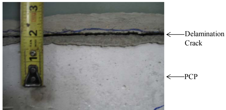
Figure 2-10: Delamination of Skewed PCP (Boswell, 2008)
